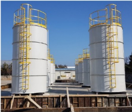
Outdoor Vertical Steel Tank
